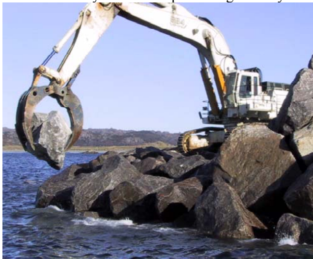
Figure 4. Construction of the Sirevåg breakwater, the 110 tonnes excavator placing class II stone
