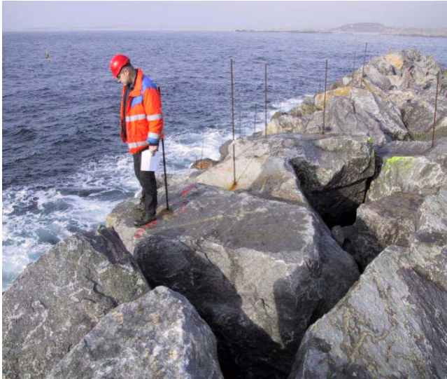
Figure 7. Inspection of the front slope of the berm of the Sirevåg breakwater, a section with class I stones.
