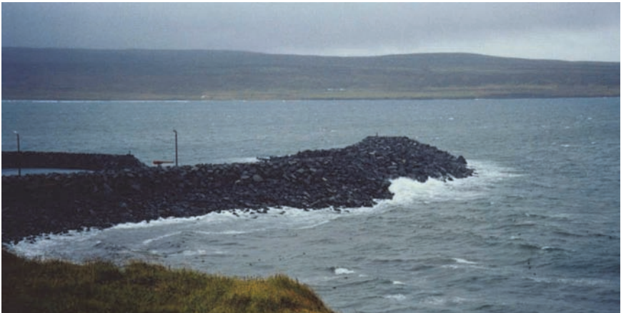
Figure 9.40. The Bakkafjordur breakwater in October 1999.
