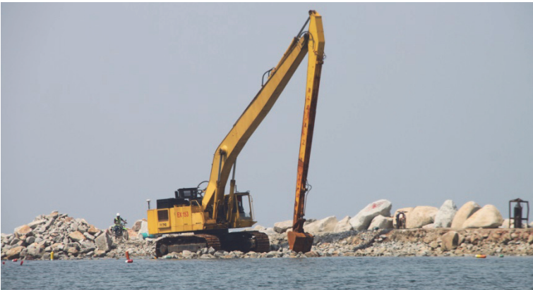
Figure 7.2. Excavator with a long boom and placed on a temporary level to place rock up to 2 t to a level of -8 m SWL.
