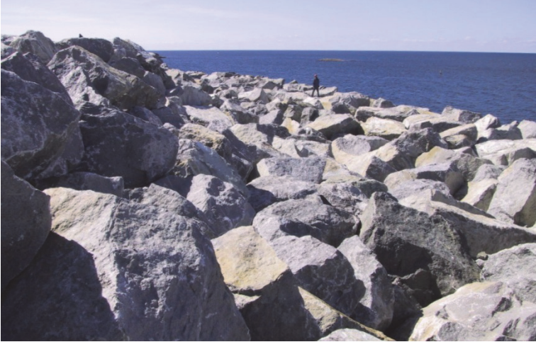
Figure 7.12. The Sirevåg berm breakwater, Norway, final inspection of the 20–30 t Class I on the berm.
