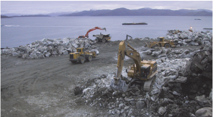
Figure 6.12. Sorting of material from the blasting pile with excavators and front loaders, at the same time loading of trucks from the stock pile. The Hammerfest project in northern Norway.
