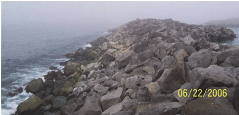
Figure 9.25. The St. George southern breakwater before the repair in 2006. The full berm width has eroded and the recession has reached the upper slope and even the crest at some locations. Wear and tear off the armourstone on the slope is evident. Courtesy of PND Engineers.
