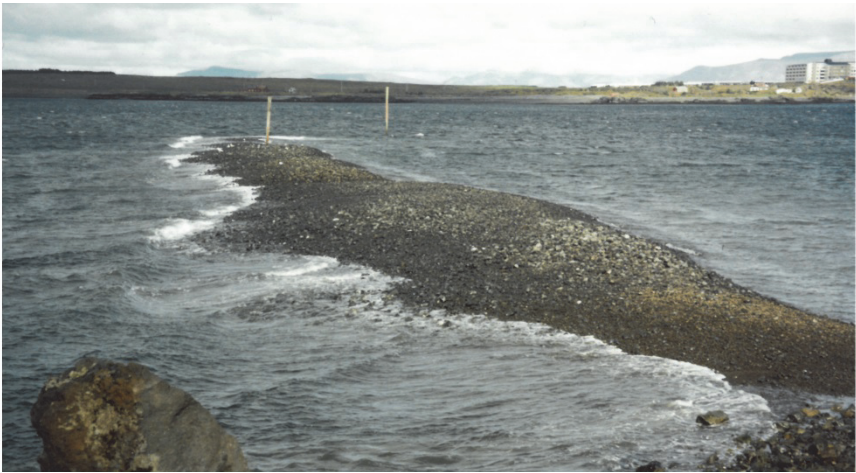
Figure 5.23. Filling of the dredged basaltic gravel on the North-South trunk of the Hafnarfjörður breakwater, finished up to about 0 to +1 m CD.
