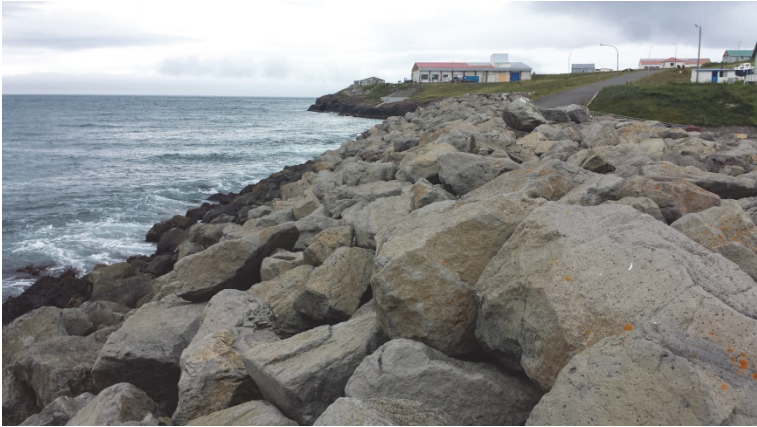
Figure 1.6. The Hofsós breakwater in 2015 which was constructed in 1983. Photo by Indridi Einarsson.
