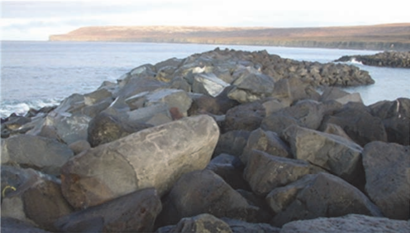
Figure 9.27. The St George southern breakwater after the repair in 2006, where freshly quarried 8–10 t rock have been added to the profile. Courtesy of PND Engineers.
