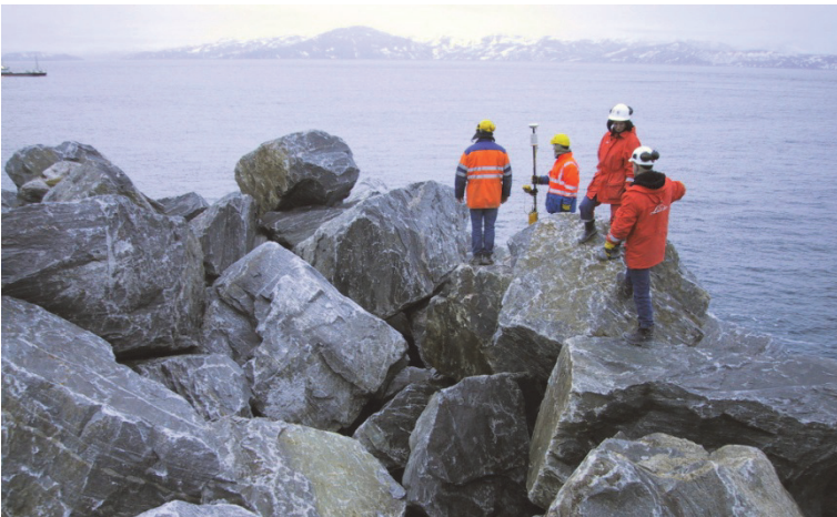
Figure 7.15. The Hammerfest breakwater, Norway, inspection survey with a GPS staff of the 20–35 t Class I stone of the unfinished berm.
