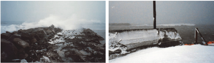
Figure 9.3. The partly constructed Dalvik breakwater during a storm event in winter 1994 to 1995. Waves breaking on the emerged breakwater, left photo, and waves breaking on the submerged mound, right photo.
