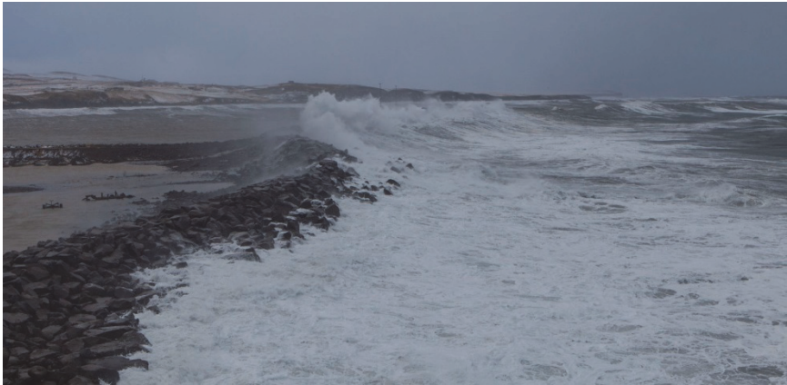
Figure 9.18. The Husavik breakwater during a storm in October 2014, waves breaking on the slope and overtopping. Photo by Gaukur Hjartarson.
