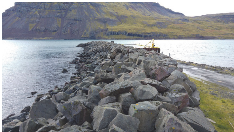
Figure 1.8. The berm breakwater at Nordurfjörður, Iceland, 30 years after construction (1984-1985). Photo by R. Kamsma.
