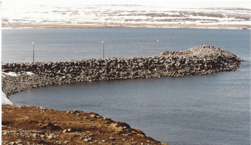
Figure 9.33. The Bakkafjordur breakwater in May 1988 with severe recession of the berm.
