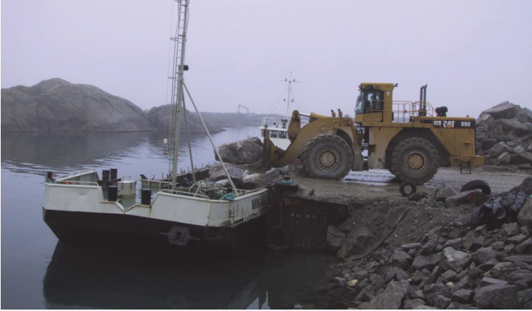
Figure 7.4. Loading a split barge with Class IV rock by a wheel loader. Sirevåg breakwater.
