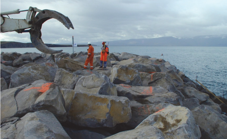
Figure 7.14. Surveying of Class I stones with a GPS staff, 16–30 t, on top of the berm before building the crest section, Husavik berm breakwater, Iceland.
