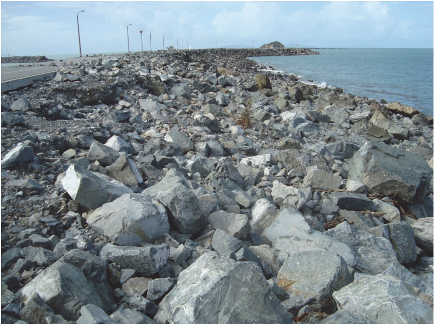
Figure 9.50. The Mackay Small Craft Harbour breakwater after the Tropical Cyclone Ului [Colleter et al. , 2011]. Photo by Gildas Colleter.
