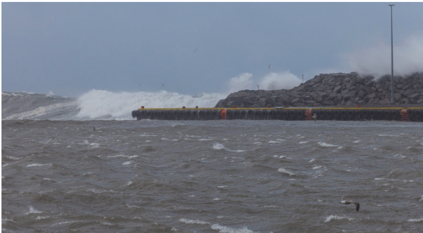
Figure 9.19. Waves breaking in front of the breakwater roundhead and overtopping the Husavik breakwater in October 2014. Photo by Gaukur Hjartarson.
