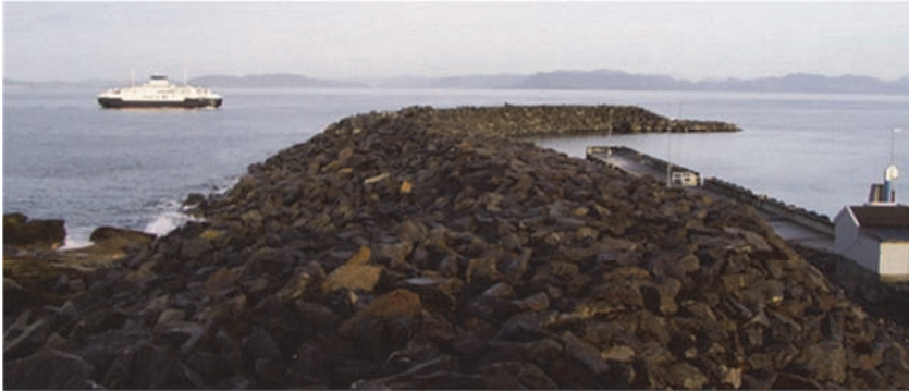
Figure 9.46 View of the Mortavika breakwater after the January 2005 storms. The berm, originally at 16 m width, is lost closest to the camera, and rocks on the top at mid-length have been rearranged and removed. Courtesy of Norwegian Public Roads Administration.
