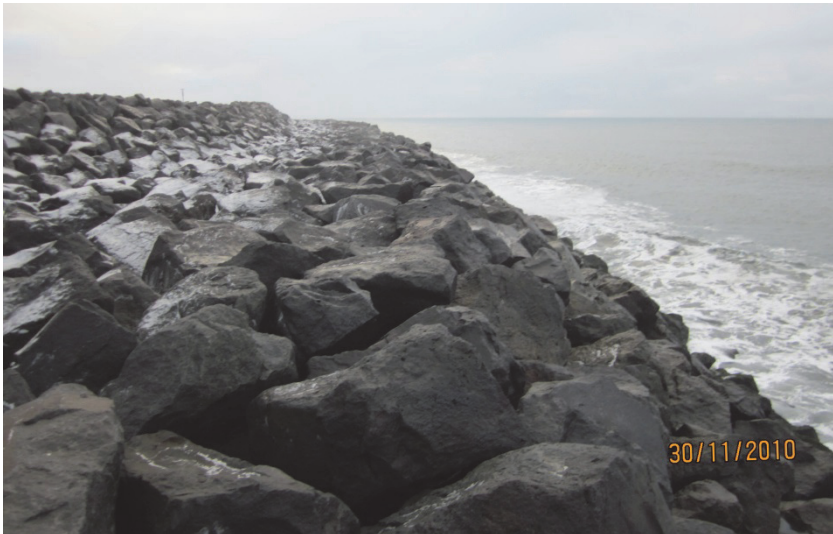
Figure 2.9. The berm of the breakwater at Landeyjahofn, where specific care was taken to place the Class I stone to enhance stability.
