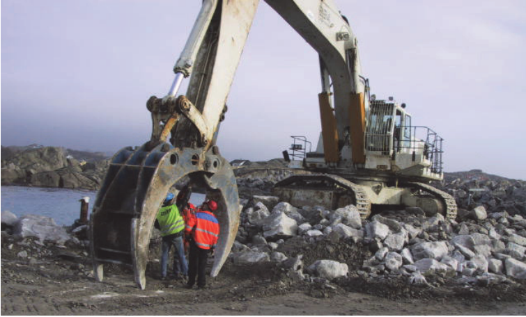
Figure 7.1. A 110 t Liebherr R984 excavator with a rock prong at the Sirevåg breakwater construction.
