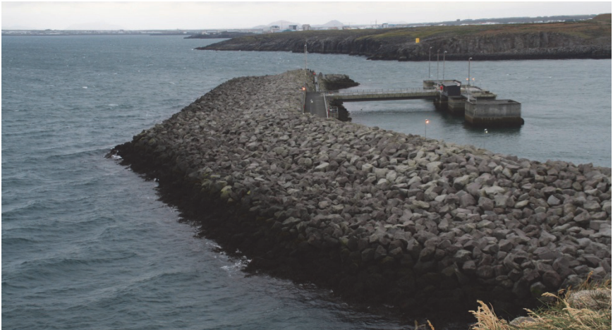
Figure 9.21. The partly reshaping mass-armoured berm breakwater at Helguvik, constructed in from 1986–1988. Picture taken in 2008.
