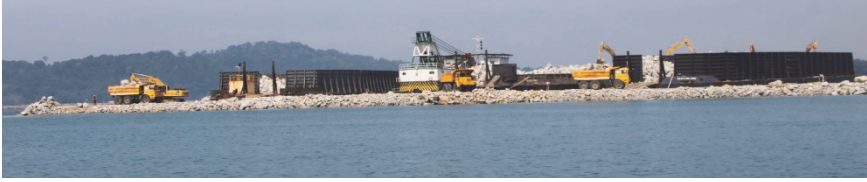
Figure 7.6. Large barges (the black boxes on the picture) importing core material, moored on the lee side of the breakwater.
