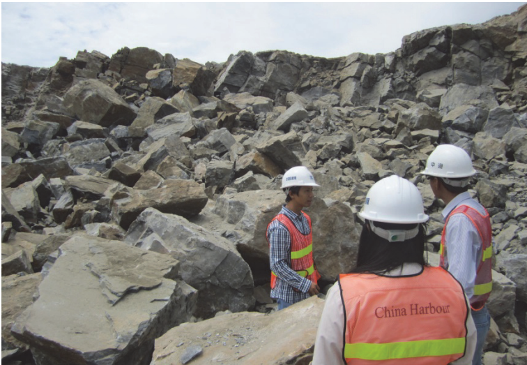
Figure 6.9. Blasting pile in the harbour excavation area of the Hambantota Port Development project, Sri Lanka.
