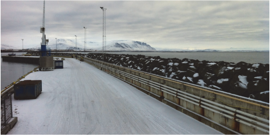
Figure 4.1. Pipelines sheltered for wave overtopping. Akranes breakwater, Iceland. Photo by Einar Guðmundsson.
