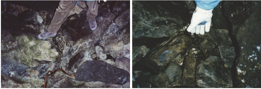
Figure 9.38. Inspection of the reshaped profile showed that deterioration of stones had caused filling and plugging of voids.
