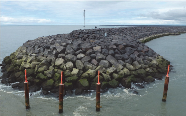
Figure 7.10. Western breakwater head at Landeyjarhöfn with special placement of Class I rock.
