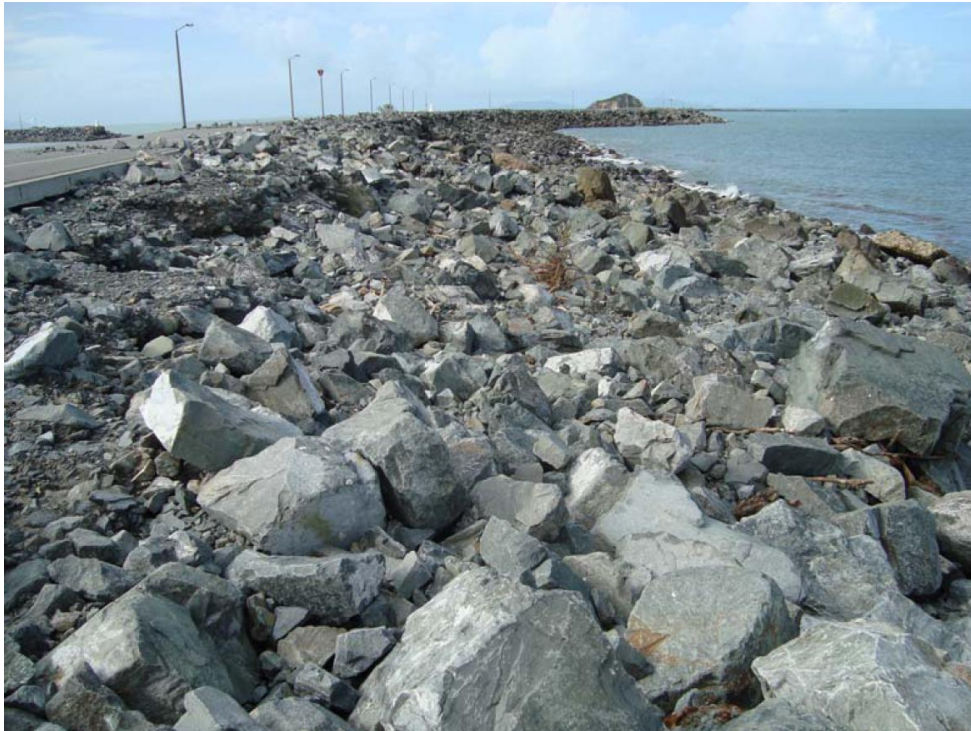
Figure 4. The Mackay Small Craft Harbour breakwater after the Tropical Cyclone Ului, from Colleter et al. (2011).
