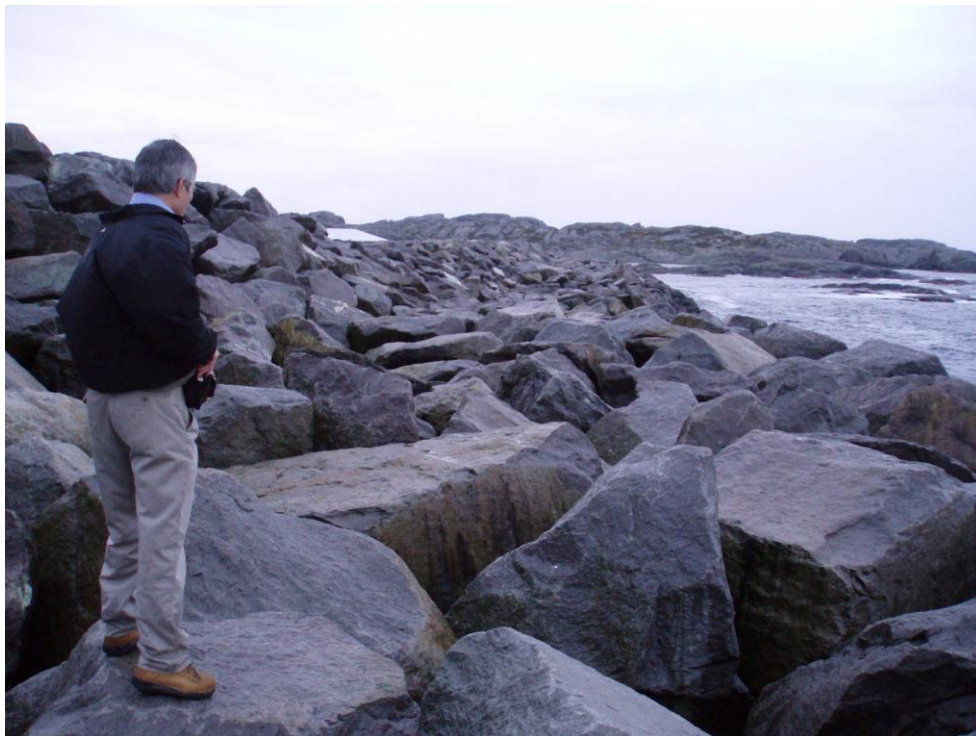
Figure 8. Inspection of the Sirevåg breakwater after being twice exposed to design wave conditions.
