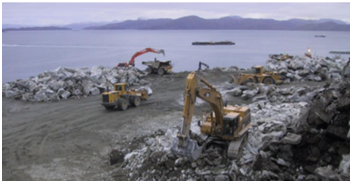
Figure 4. Sorting of material from the blasting pile with excavators and front loaders, loading of truck from the stock pile. The Hammerfest project.
