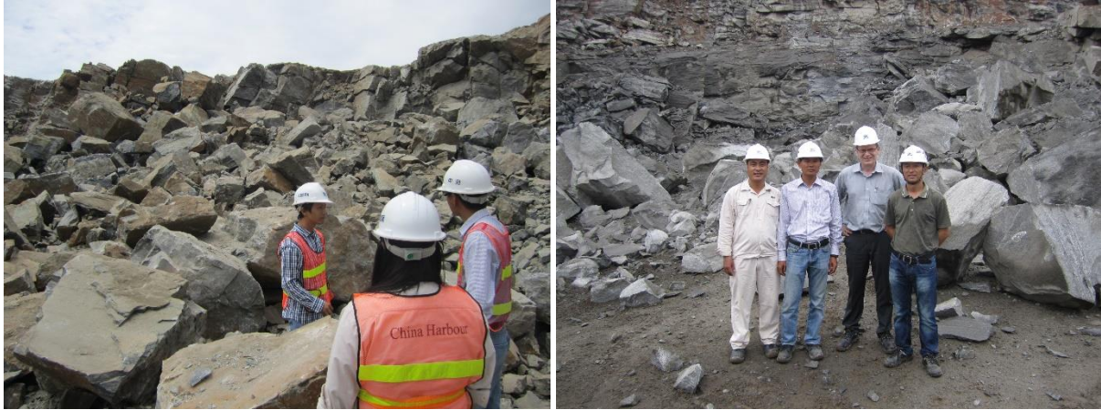
Figure 5: Hambantota Port Development project, the contractor's team examining the blasting pile after test blasting in the harbour basin area.
